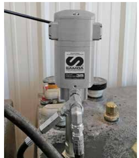
Tank mounted pump
