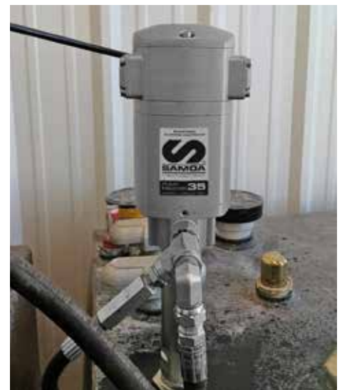
Tank mounted pump
